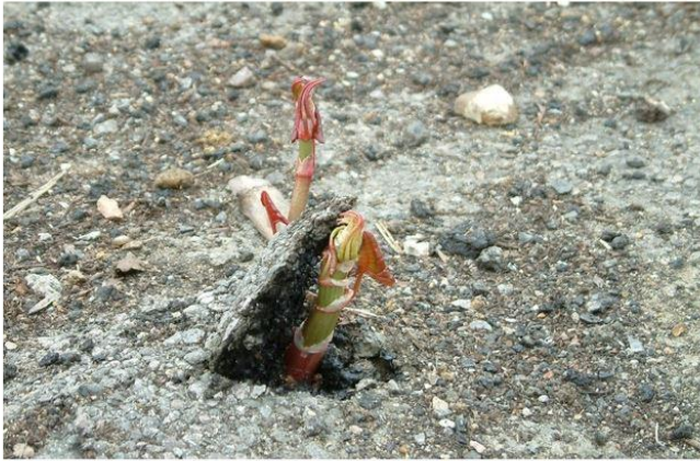
Japanese knotweed breaking through concrete © GB NNSS
