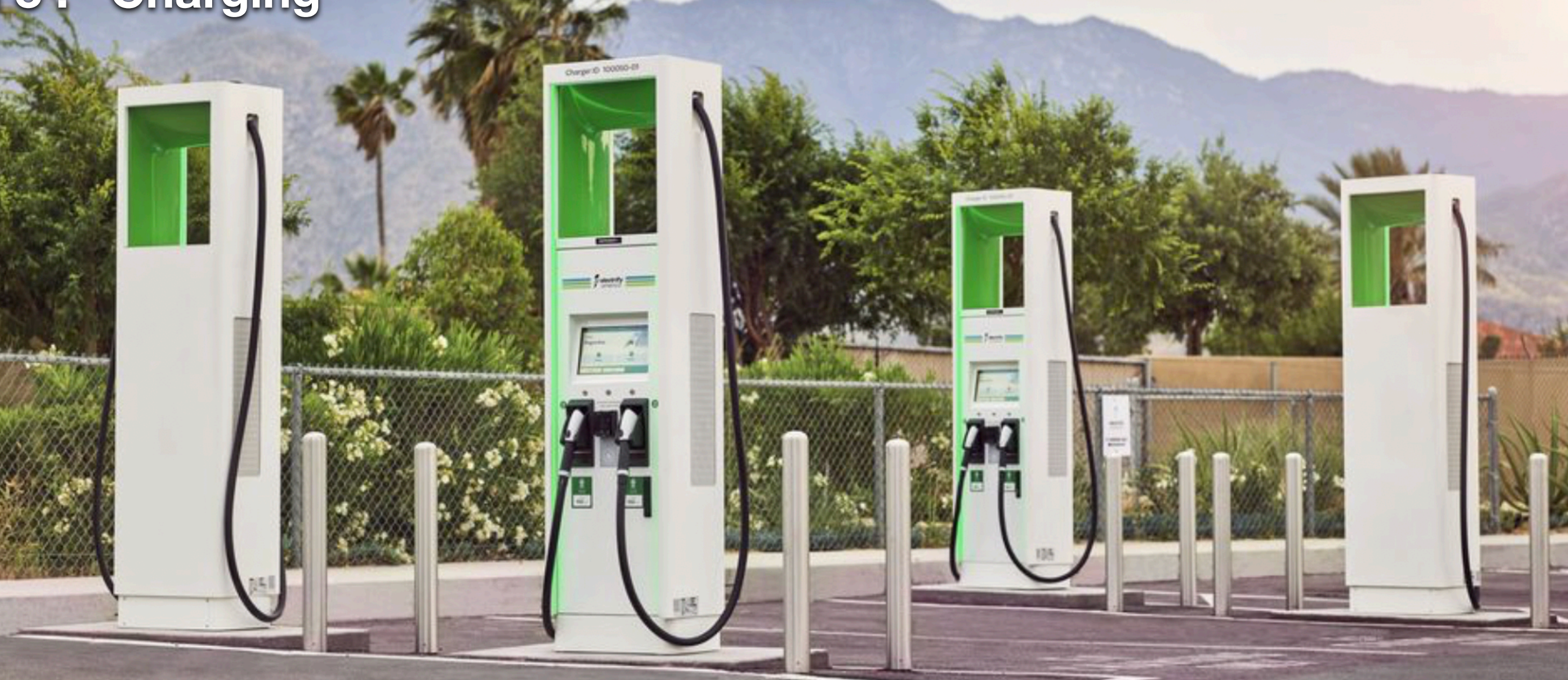
Electrify America station
