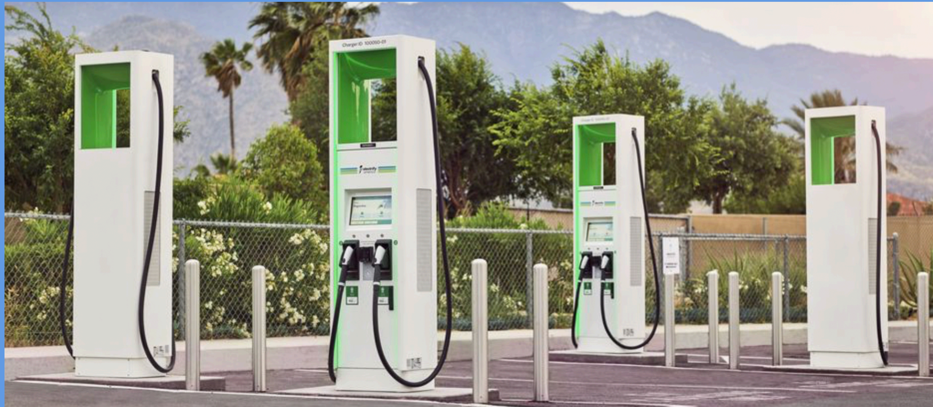
Electrify America station
